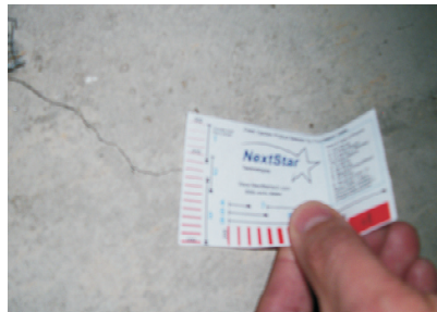
Place next to Crack to measure size
